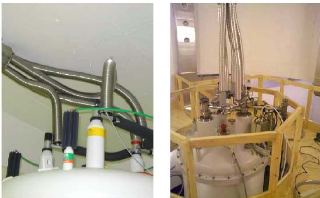
Figure 8.3: Emergency Quench Pipes
