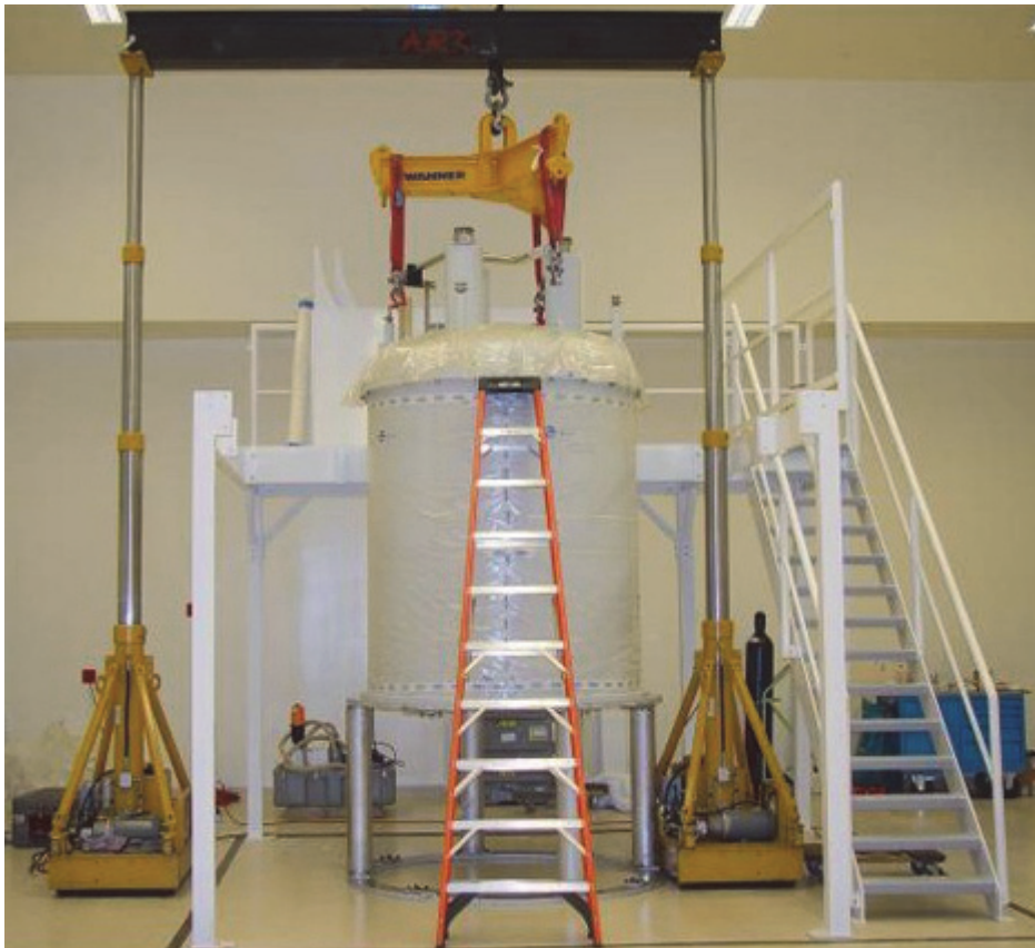
Figure 5.1: Hydraulic Gantry for Lifting the Magnet Inside the Magnet Room
