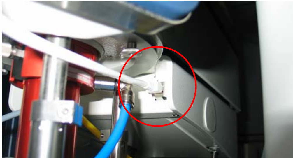
Figure 5.19 Location of the Ethernet Cable
