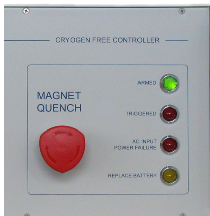
Figure 5.15: Emergency button MAGNET QUENCH on the BCFC front panel
