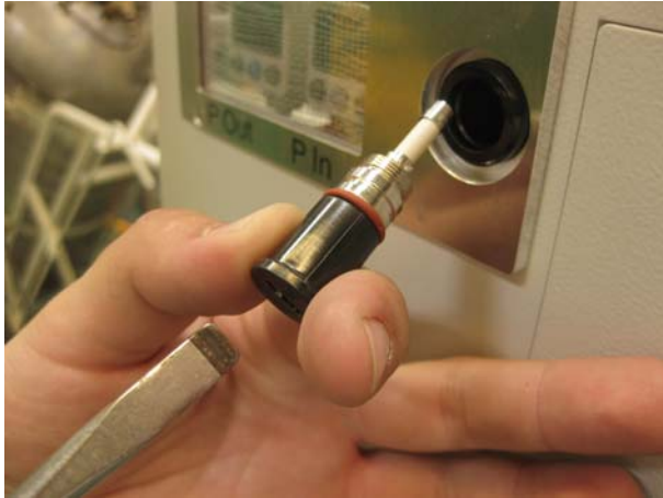
Figure 8.6: Cryocooler Controller Fuse Holder
