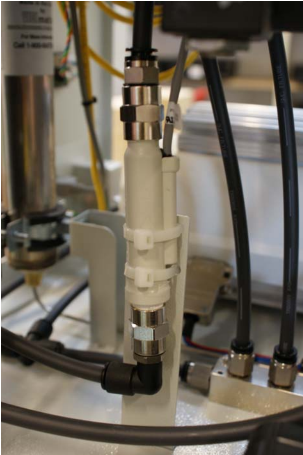
Figure 4.6: Coolant Flow Switch
