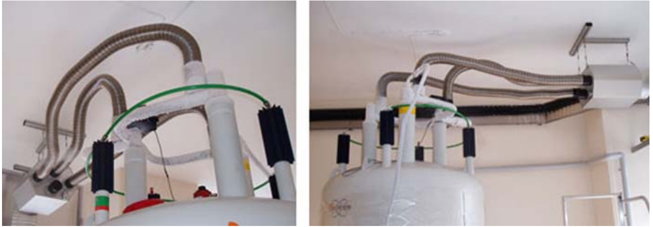
Figure 8.2: Emergency Quench Pipes
