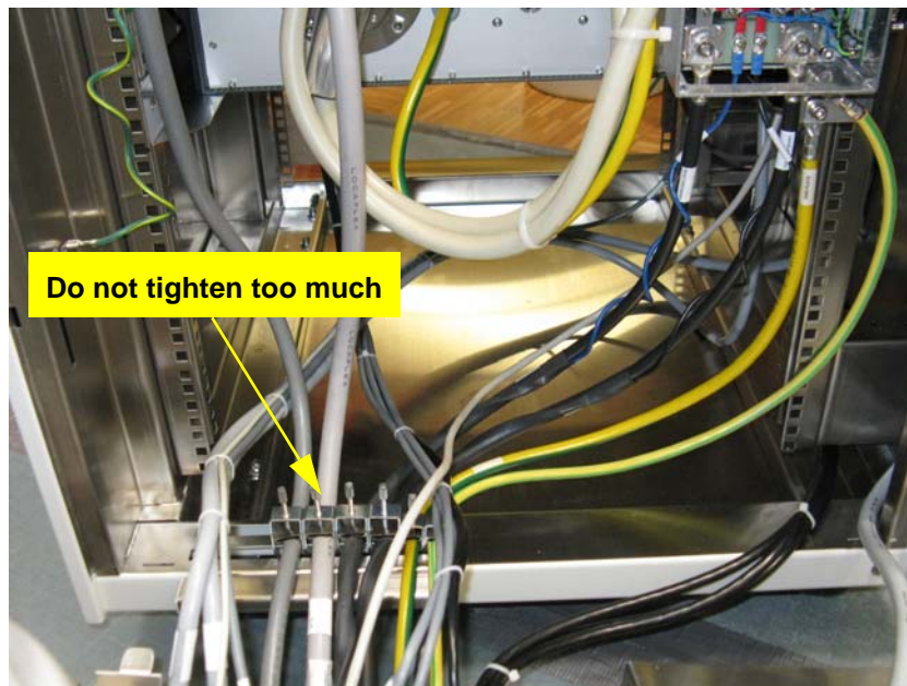
Figure 7.45 Strain relief at console entry
