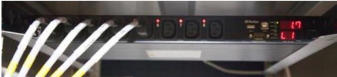
Figure 3.3: The Power Distribution Unit
