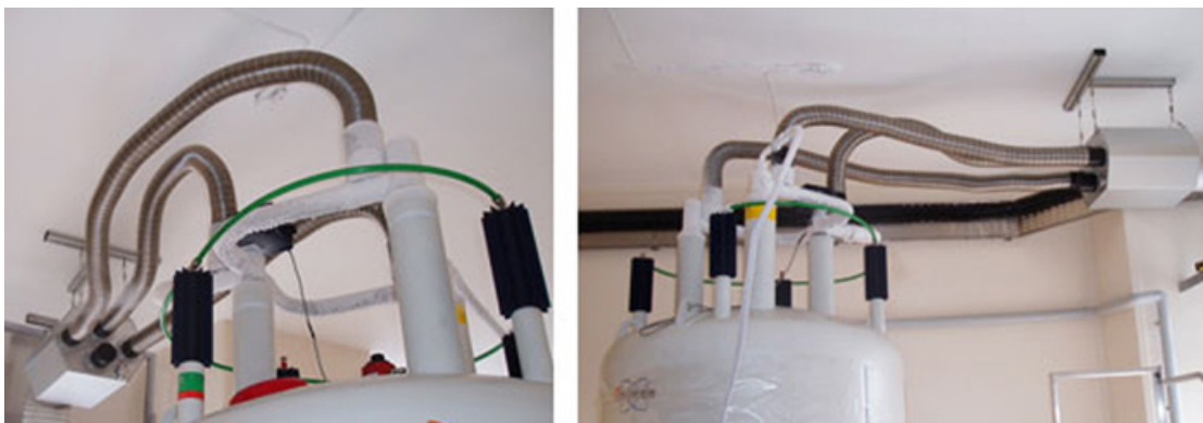
Figure 8.4: Emergency Quench Pipes
