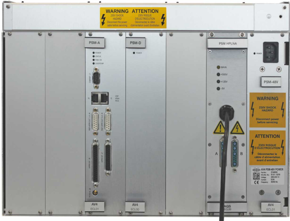
Figure 7.1: Overview AV4 Power Supply Modules
